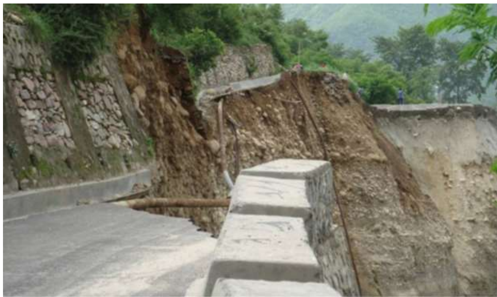
Damaged approach road, falling retaining wall and water supply line as on 27-06-2013
